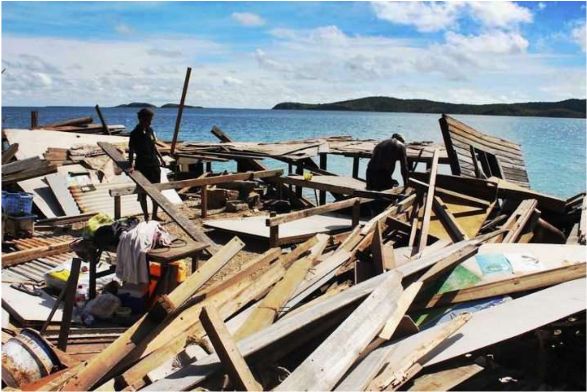
Image 5: Many Paga Hill residents lost both their home and furnishings in the demolition. Photo courtesy of Jeffrey Feeger.
