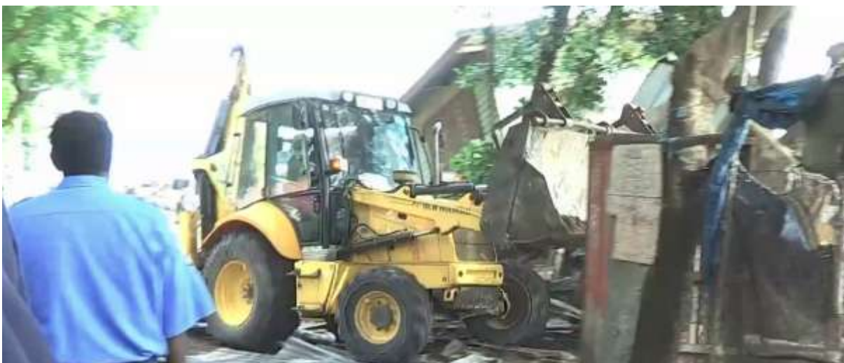
Image 4: A bulldozer demolishes homes at Paga Hill. Image courtesy of Media Stockade.
