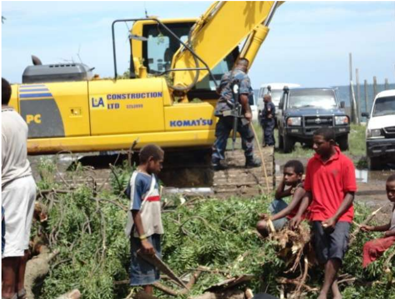
Image 6: An excavator hired by PHDC for the May 12 demolition manned by an armed police officer
